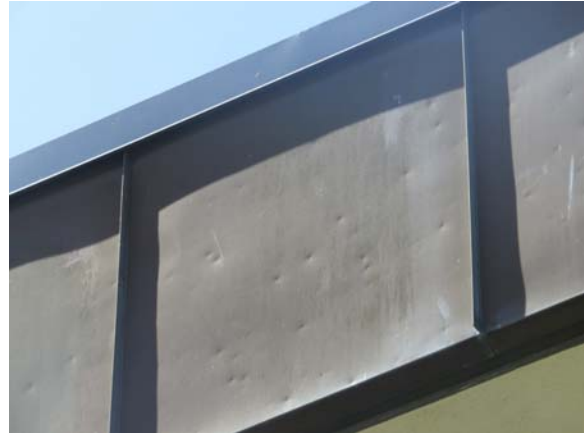
Figure 4: Cosmetic damage or more?
